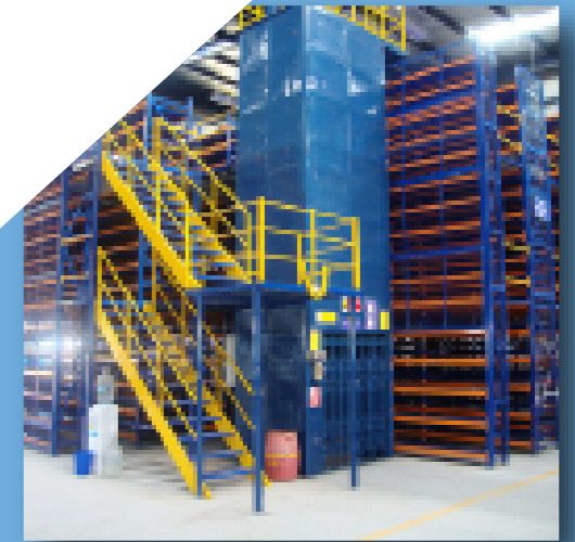
Mezzanine and Multi-tier Rack ▲
